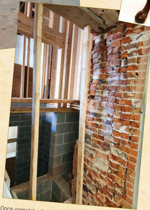
Once complete, the elevator will connect Hotel Garber with the Farmers and Merchants Bank, bridging the brick wall that is nearly three feet thick.
