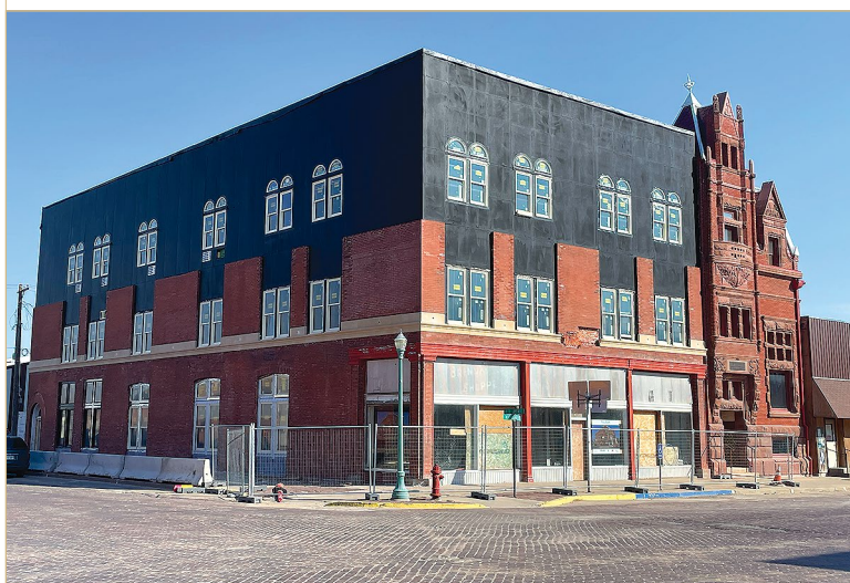
Recent facade work included replacement of brick and installation of precast stone below second floor windows.
