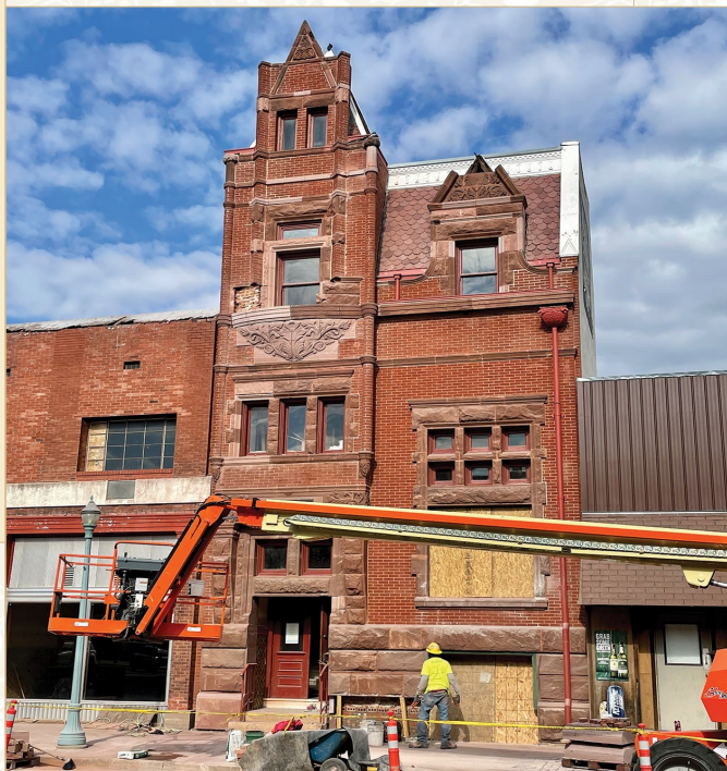
The Farmers and Merchants Bank has been receiving a sensitive historic facelift and much attention inside.
