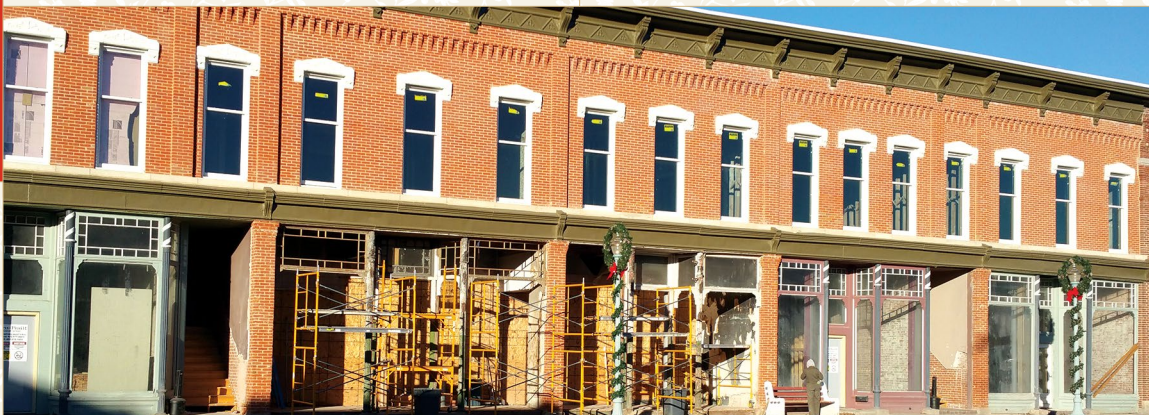
Front façade restoration begins on first floor of the historic Moon Block.
