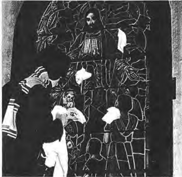
Wadded rags aren't very pretty, but they work to stop blizzard-driven snow from sifting through the small holes in the window over the altar of the Grace Episcopal Church.—Photo by John English.
