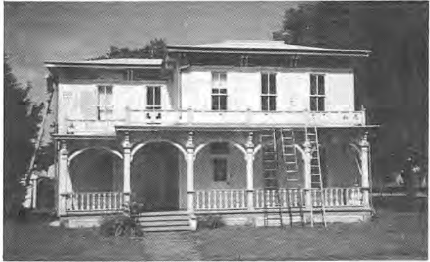
The Harling House (My Ántonia) owned by Bernard and Nancy Picchi of Bernardsville, New Jersey, received another boost toward restoration this summer when the Picchi's had the house painted its original colors.
