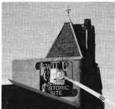
Work in progress — the new sign high atop the Willa Cather State Historic Site clearly marks the Museum Building (The Farmers' and Merchants' Bank Building).
